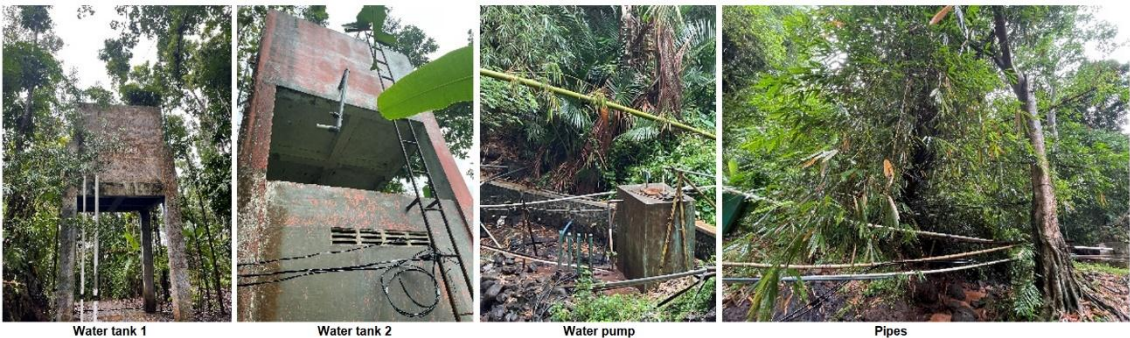
Fig. 3. Water production unit condition
