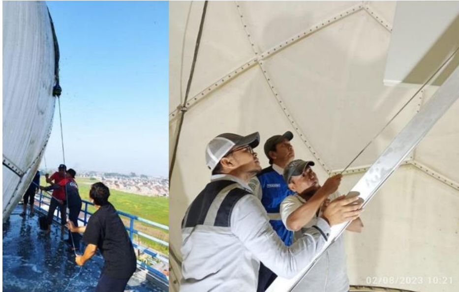
Figure 2. Weather radar maintenance
