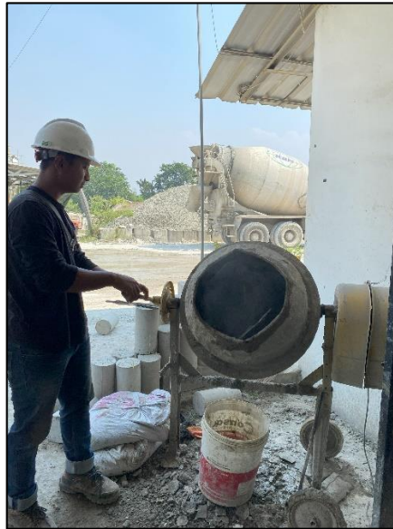
Fig.4. Concrete mixer machine
