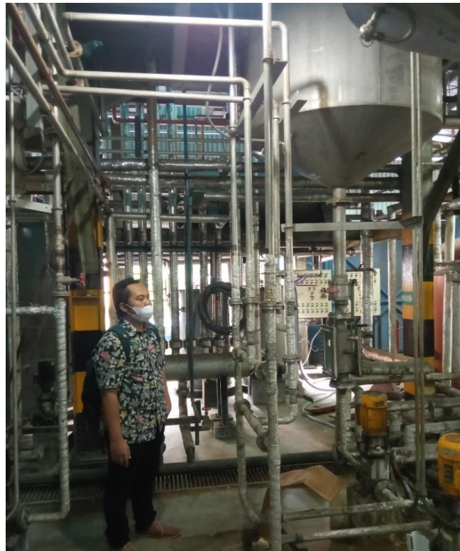
Fig. 1. Biodiesel production transesterification reactor tank
