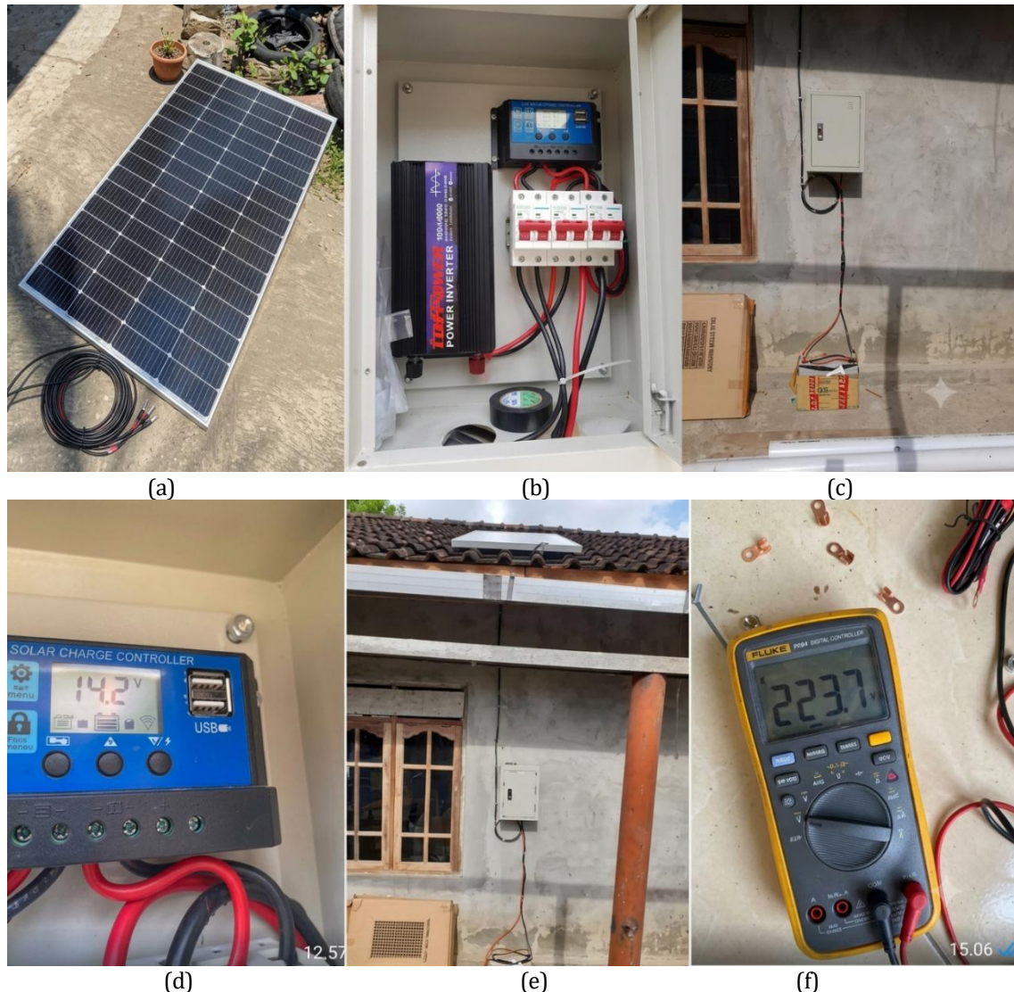
Fig. 4. (a) 300 wp panel, (b) control panel installation (solar charger controller, MCB, Inverter), (c), (d), (e) Solar Panel Installation, Control Panel with Battery, (f) 223,7 Volt output result
