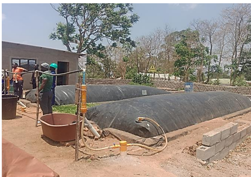
Fig. 4. Tsangano Biogas Plant in Ntcheu District
