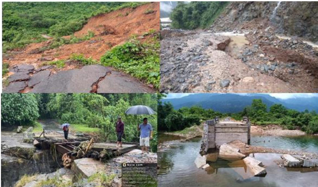
Figure 3B. Specimen photographs of eroded section of roads and bridges (Sources: DDMA, SWKH)
