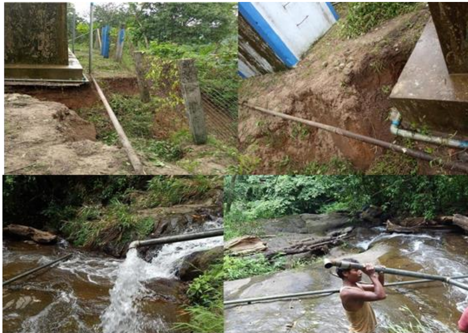
Figure 3D. Specimen photographs of eroded section of gravity main pipe lines (Sources: DDMA, SWKH)
