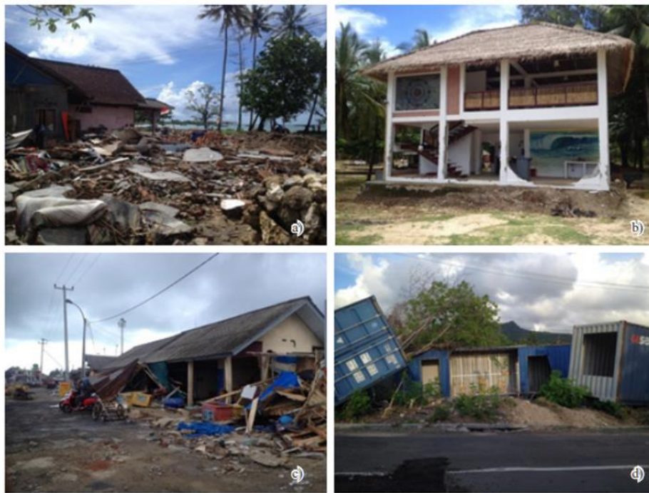
Figure 1. A densely populated residential area in Kertajaya Village, Sumur, Pandeglang, Banten which was destroyed by the tsunami on December 22, 2018.
